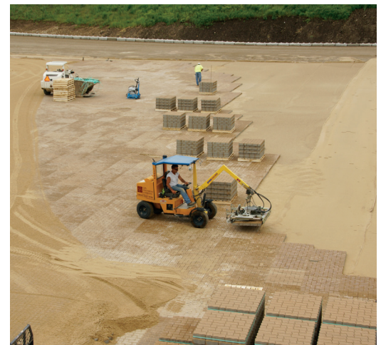
Mechanical installation of Renewable Pavers™ manufactured by County Materials Corp., allow for large scale projects such as this one to be done in a fraction of the time it would take to be hand laid.
